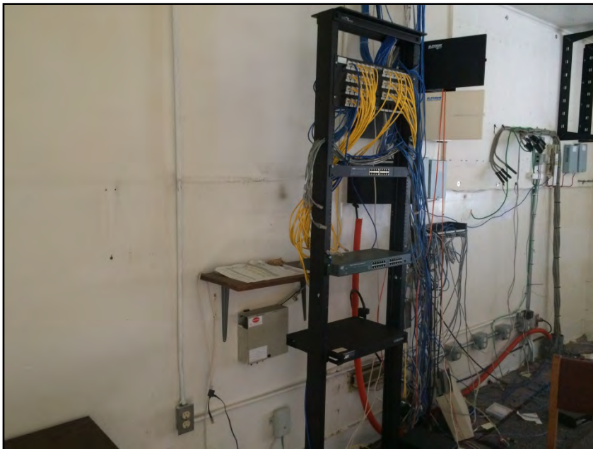
Photograph No. 38: View of a communications closet.
