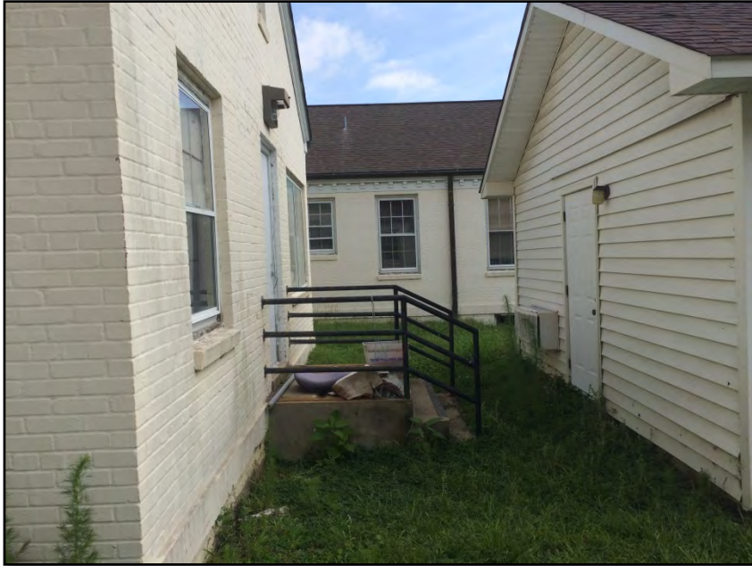
Photograph No. 7: View of the space between the shed and the main building.
