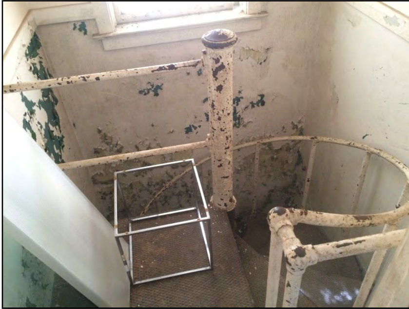
Photograph No. 41: View of the steel spiral stairs that leads to the basement.
