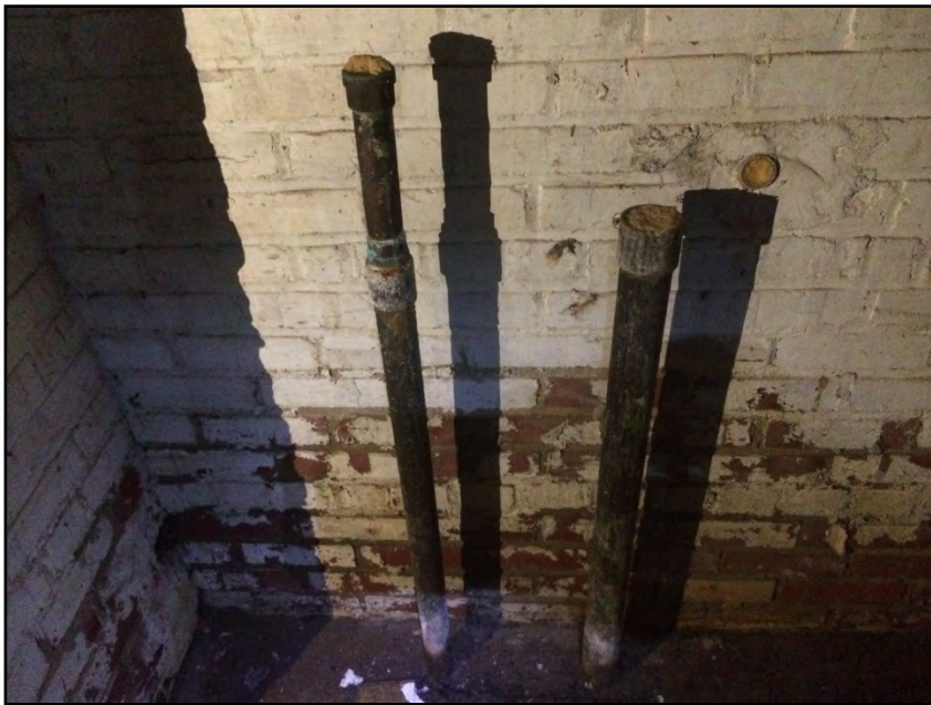
Photograph No. 44: View of the vent and fill pipes to the former UST.
