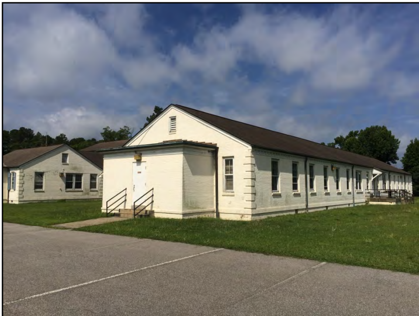
Photograph No. 10: Additional view of the end of the northeast wing showing the north facing (rear) elevation.
