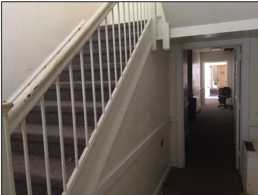
Photograph No. 34: View of the stairs that lead to the upstairs nurse's quarters.
