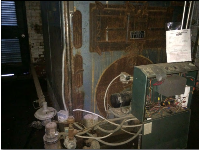
Photograph No. 43: View of the boiler.
