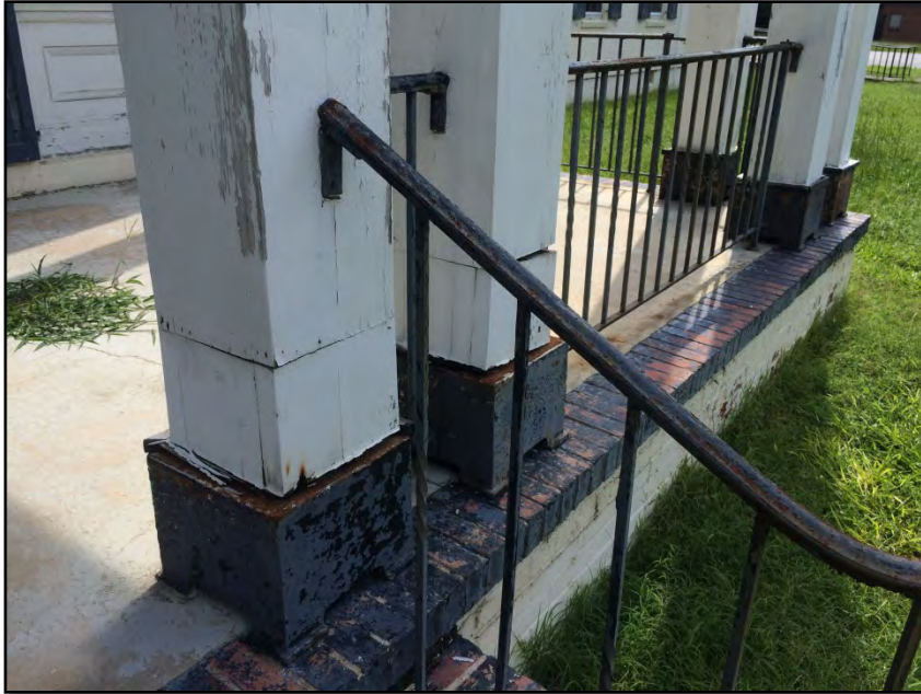
Photograph No. 21: View of the bottom of the front porch columns and railing.
